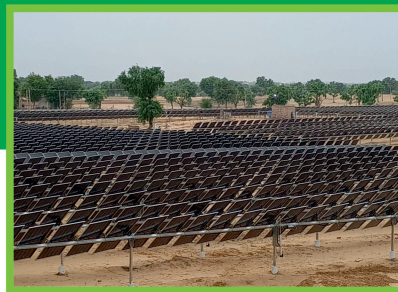
ANGIRA LIME INDUSTRY, 2.52 MW (Churu) (Single Axis Tracker Structure)
