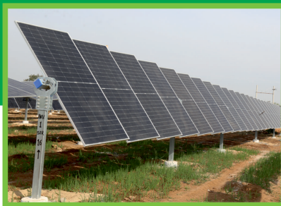
SUNBEAT ENTERPRISES, 1.5 MW (Chittorgarh) (Single Axis Tracker Structure)
